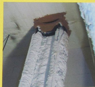
After the fire test of Promapaint SC, Pavus a.s., report No. Pr-06-2.019
