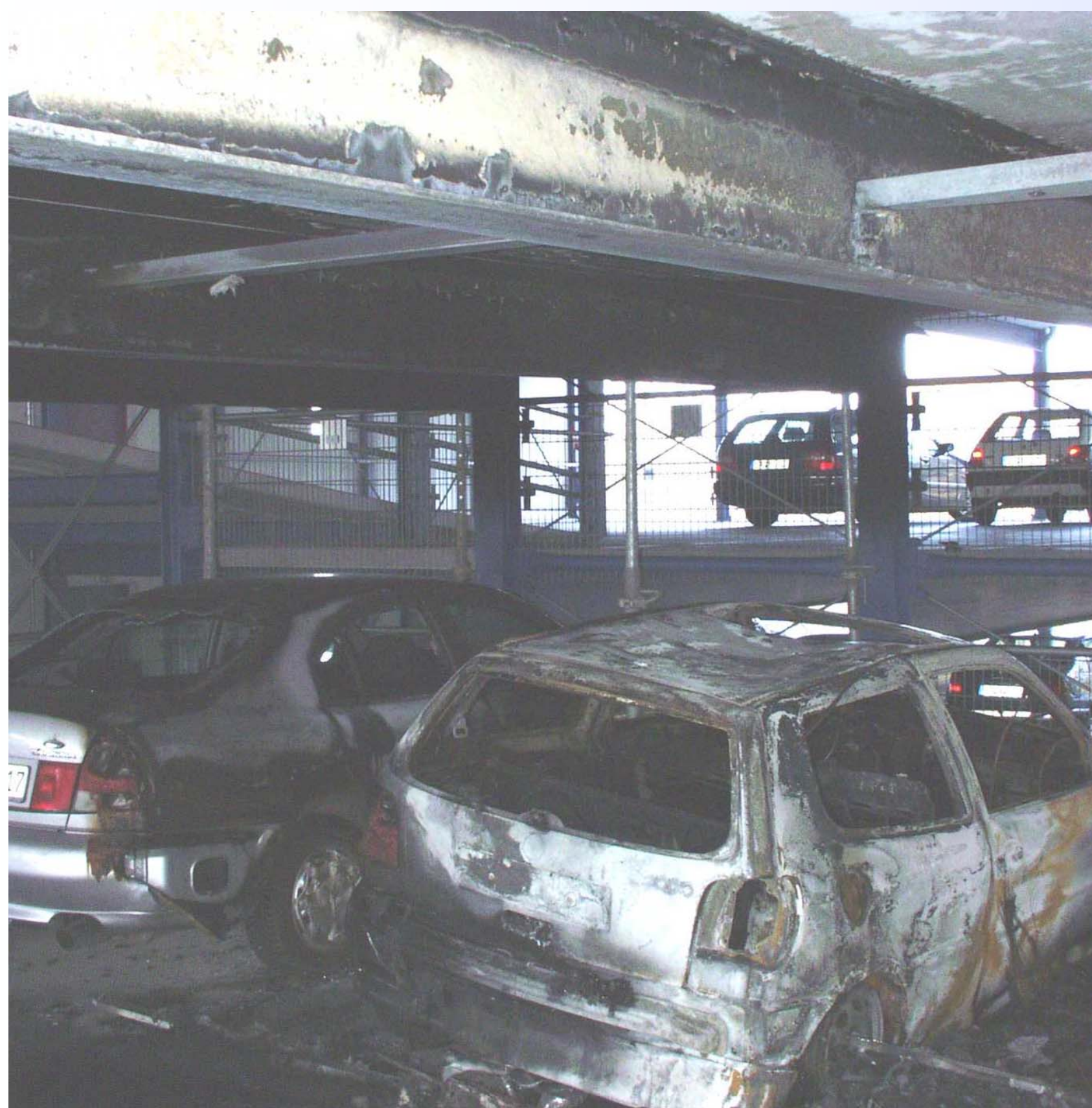
Fig. 1: Cars and composite beam after fire in car park
