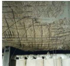
Figure 1 Explosive Spalling of ceiling slab (Bailey 2000)
