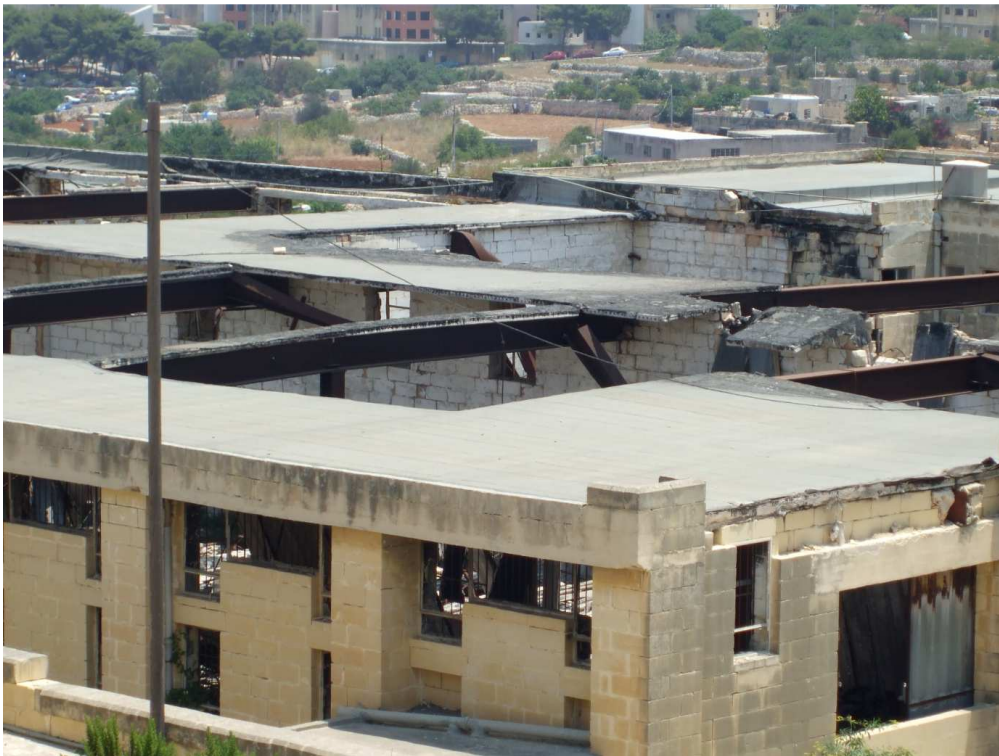
Fig. 1 Damaged load-bearing masonry building in Malta exposed to fire
