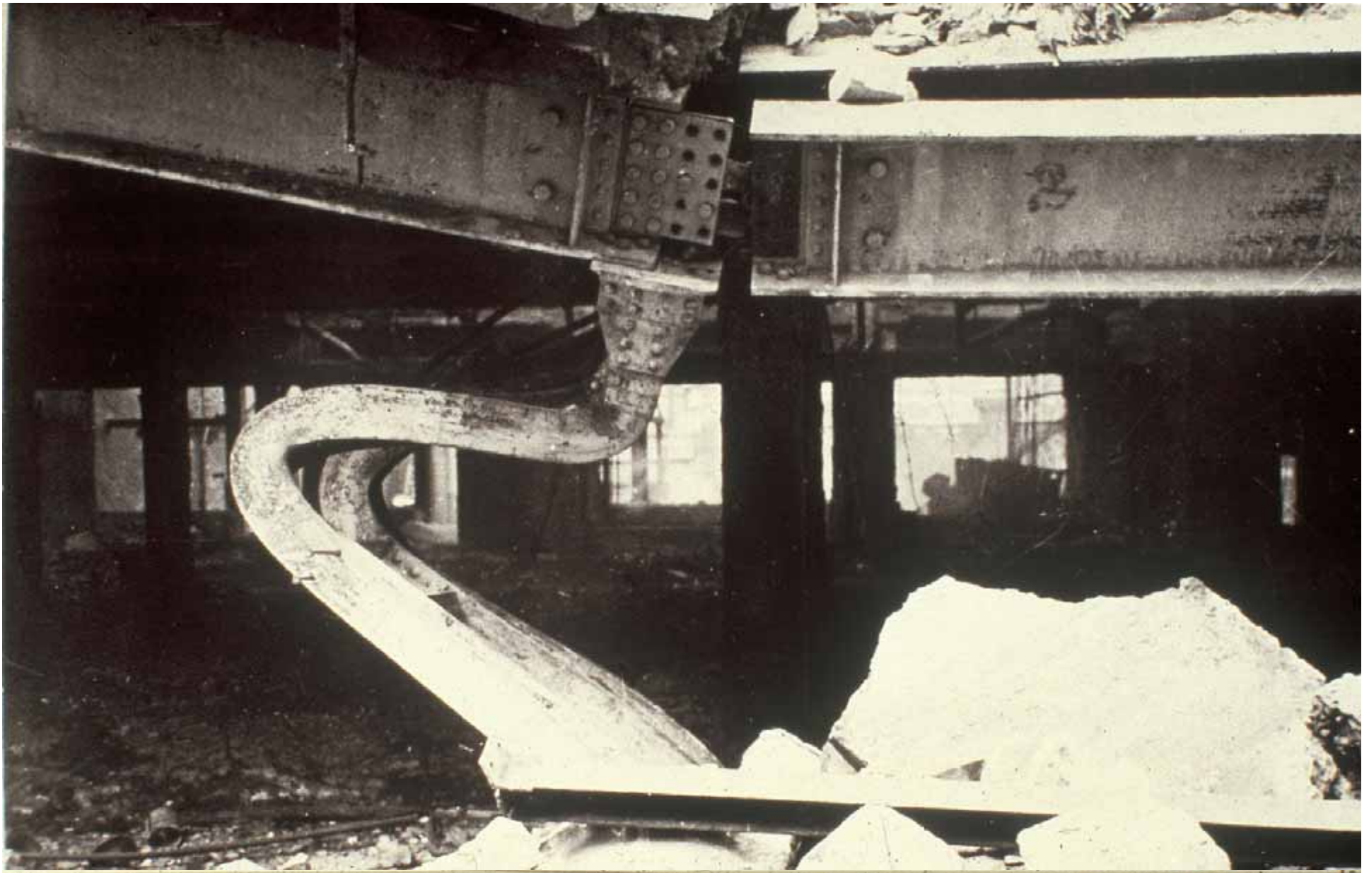
Resulting connection failure
