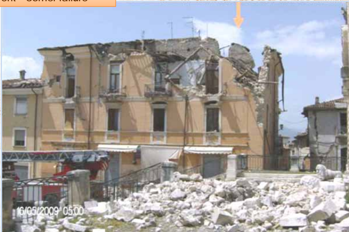
OLD Palace after seismic event - corner failure -
