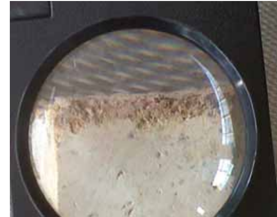
Thickness degraded - 2,66cm
