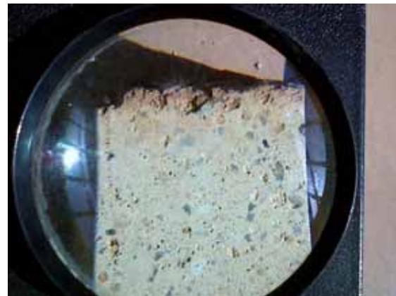
Thickness degraded - 4,11cm
